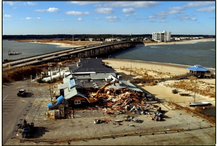
Four-story condominiums are now planned for the property at the base of the Lesner Bridge. This photo shows the 2005 demolition of the Duck-In restaurant. (Stephen M. Katz, Virginian-Pilot file photo)
